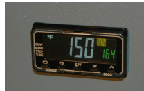
Digital Temp controller mounted on face of electric box
